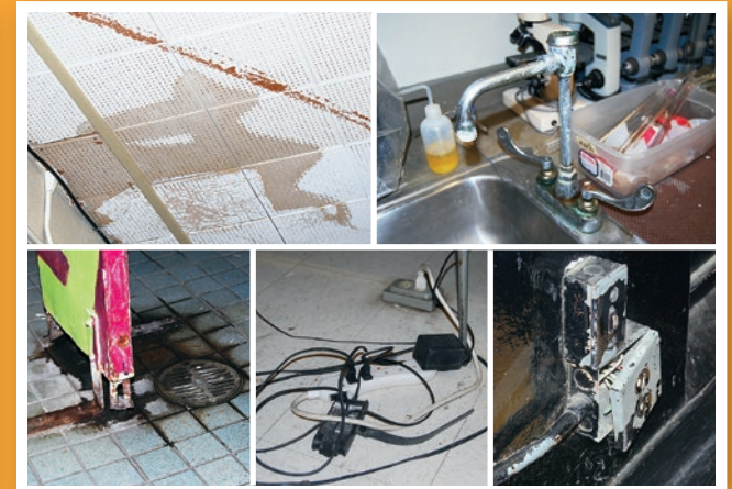
▲ Repair / replace leaky roofs, old rusty plumbing, outdated electrical systems.
