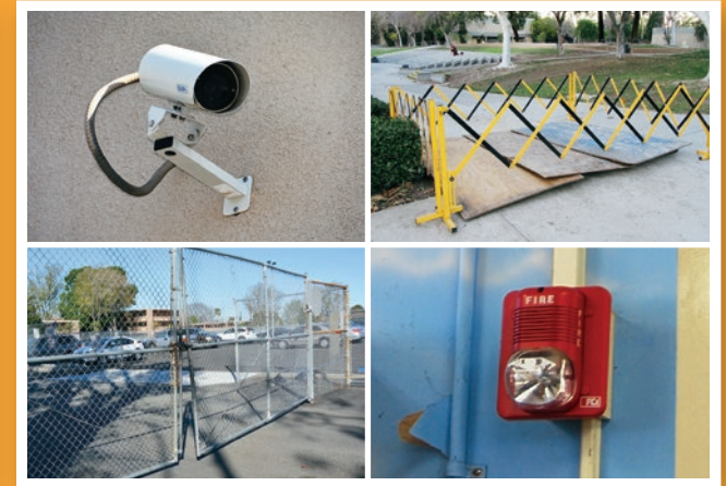
▲ Upgrade safety and security; add cameras and safety equipment; remove hazards.
